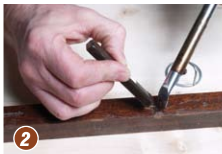
2 A heated spatula is used to melt a filler stick of the correct colour. This can then be dripped into the hole and the spatula applied to smooth it out
